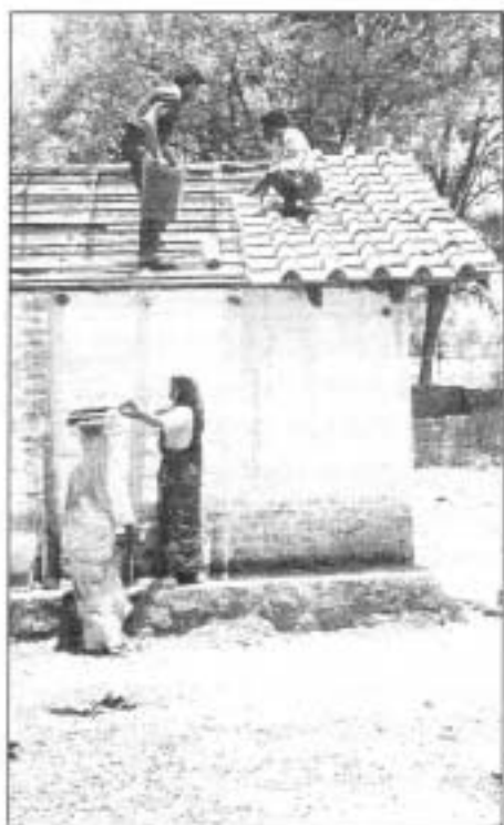
The new roof allows children to study under the monsoon - not in it!
