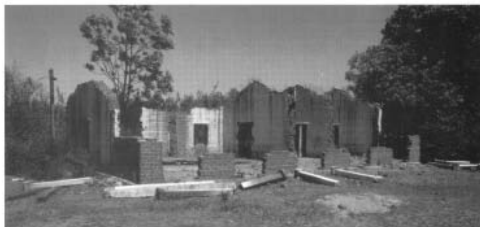
Classrooms badly in need of attention before the monsoons
